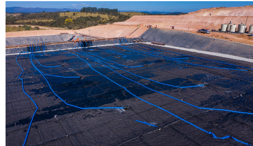
Overview of bags used for storage and dehydration of tailings dredging. The water drained from these bags is pumped to ETAF and returns clean to the Paraopeba river. Photo: Vale Archive.
