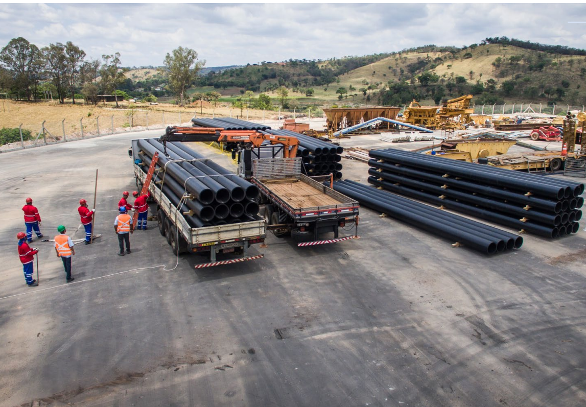
Beginning of the pipeline works in Pará de Minas (MG). Photo: Vale Archive.
