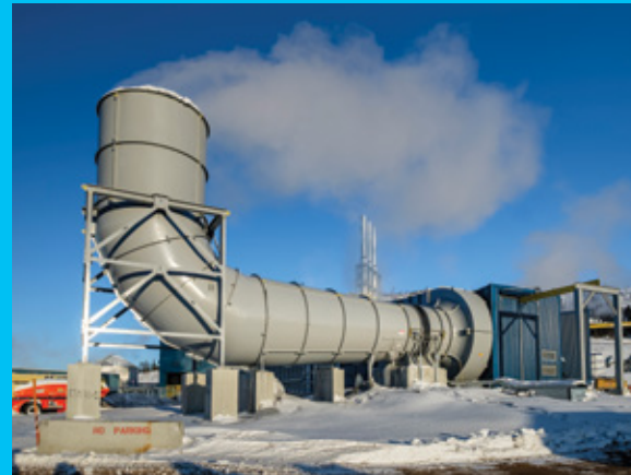
VBME Project Update: Reid Brook Underground Mine Return Air Raise Fans.
