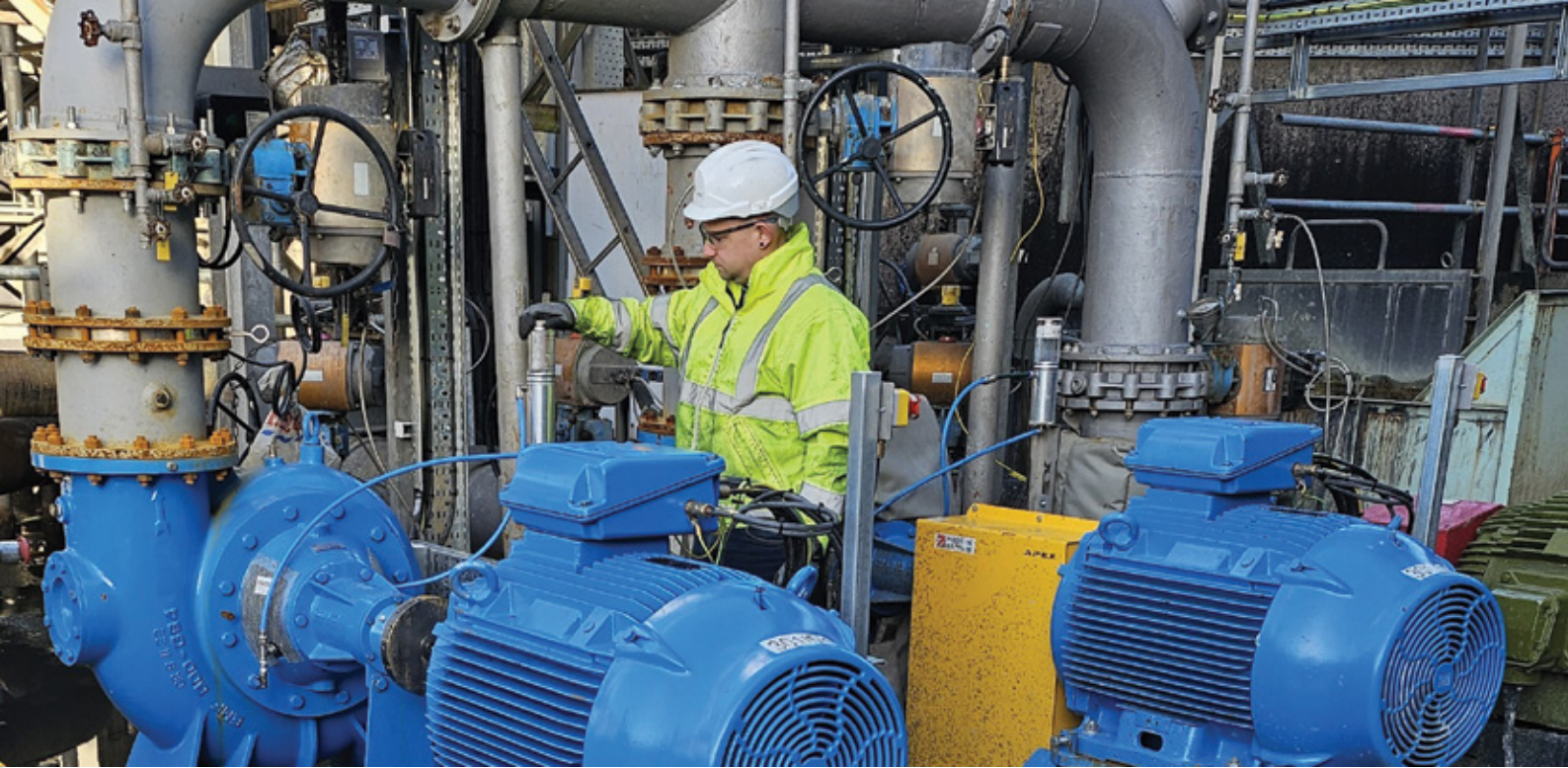
Mark Fish, Senior Coordinator of Production, checks the new VSD pumps in our Effluent Plant.
