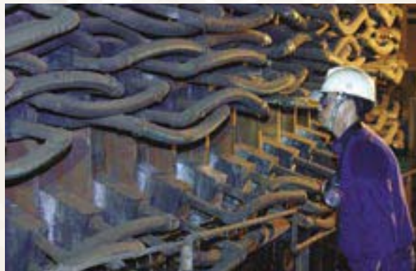
Sistem pendingin sisi luar dibangun pada Tanur No. 2. Sidewall coolers were reinforced on Furnace No. 2.
