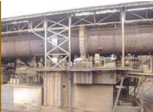
Kami memasang Variable Speed Drive pada Tanur Pereduksi No. 2. We installed a Variable Speed Drive on Reduction Kiln No. 2.
