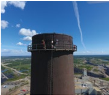
The top of the Smelter stack is being capped as part of the decommissioning process.
