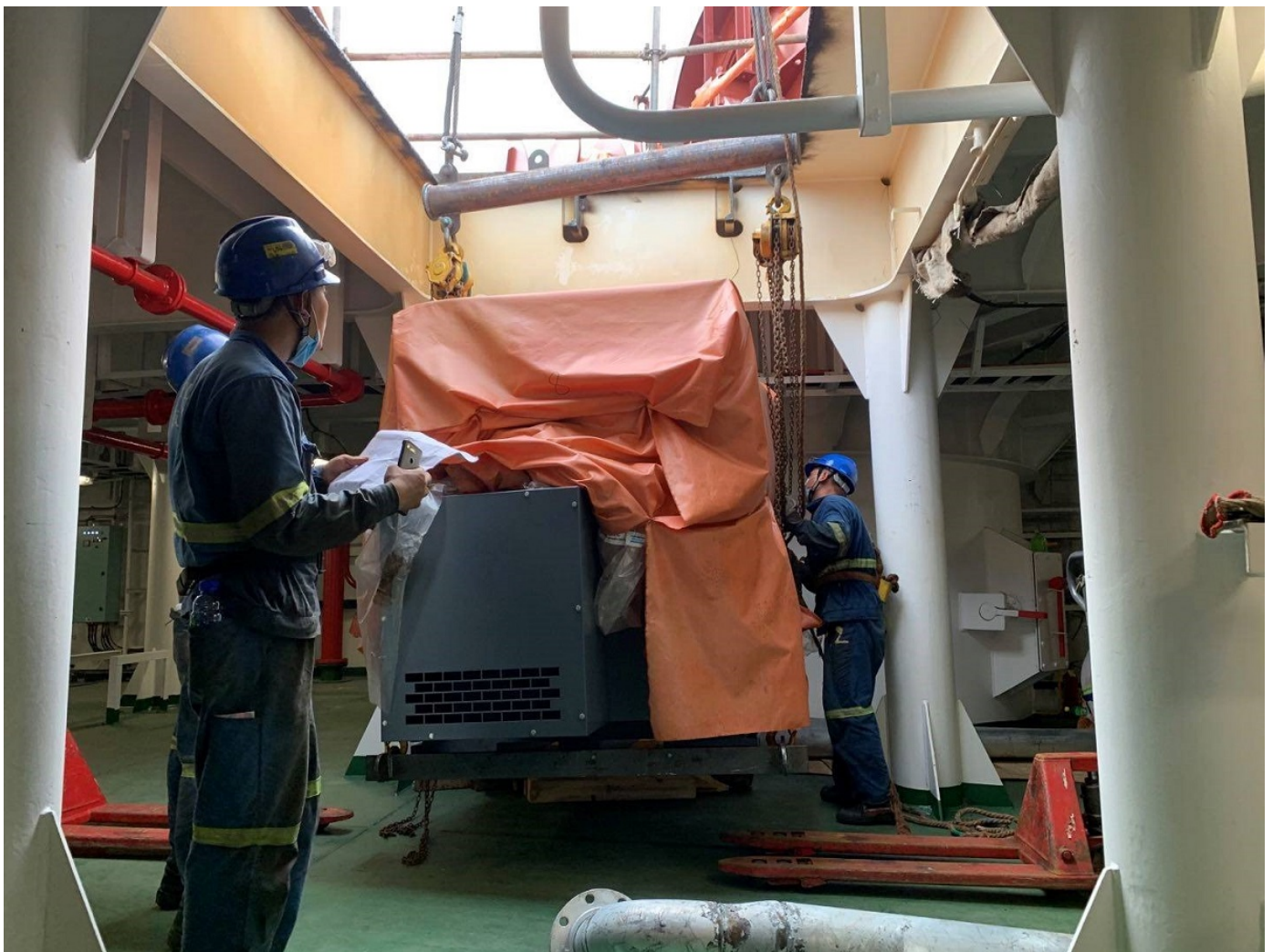
Workers receive one of ten compressors installed on the ship's deck that send air to devices positioned under the ship
